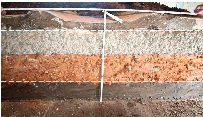
Figure 1: Typical cross section of pavements damaged by rutting.
